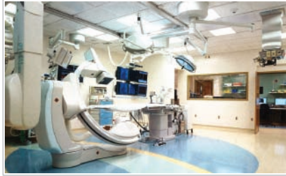
A.I. DuPont Hospital Hybrid Cath Lab, Delaware ▲
